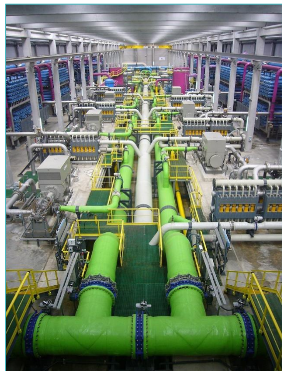
Figure 24: Reverse osmosis desalination plant
